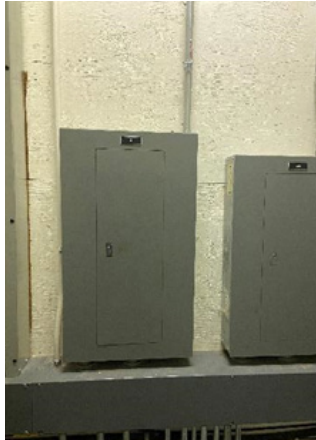
Older Electrical Panels
