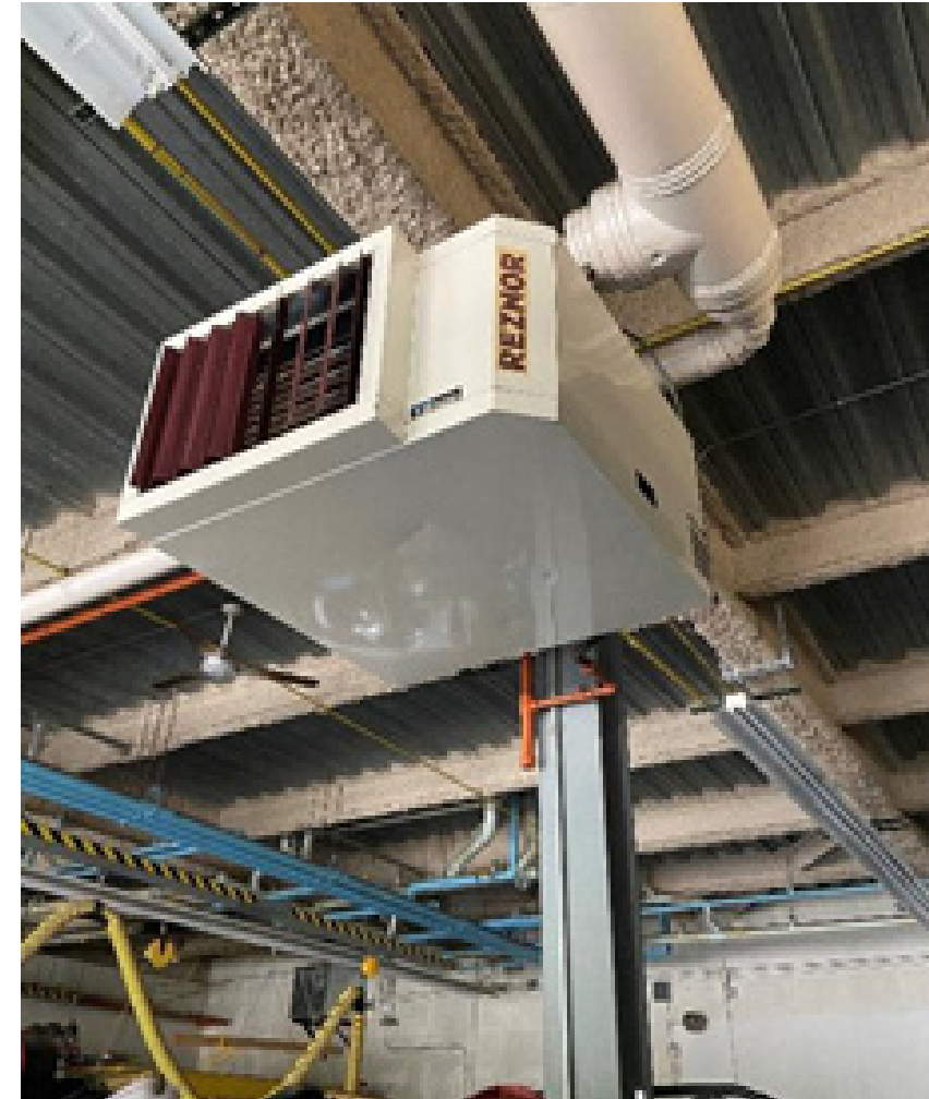
Gas Fired Unit Furnace
