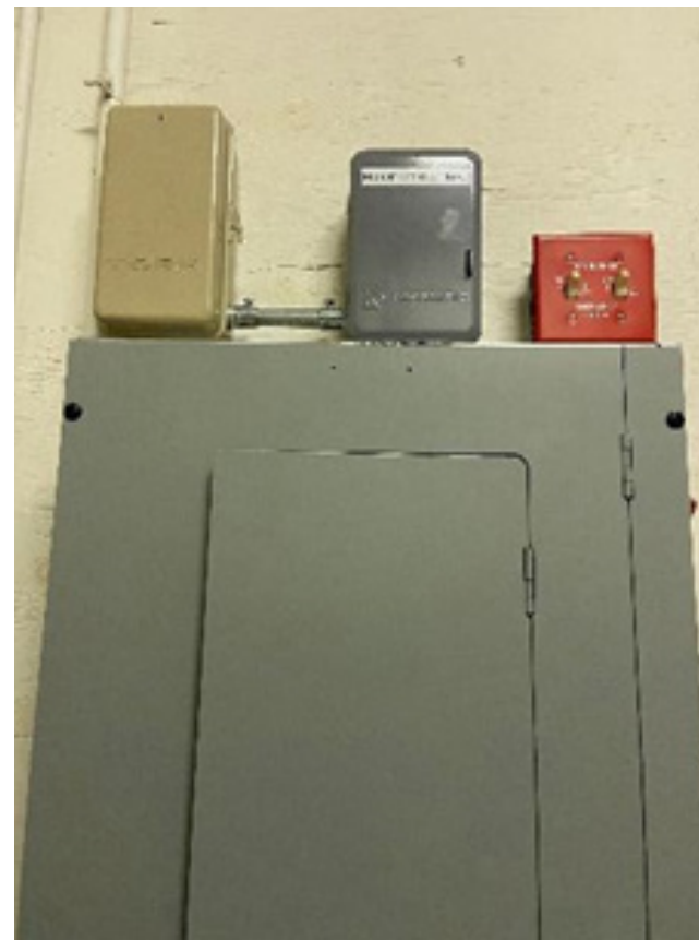
Newer Electrical Panel
