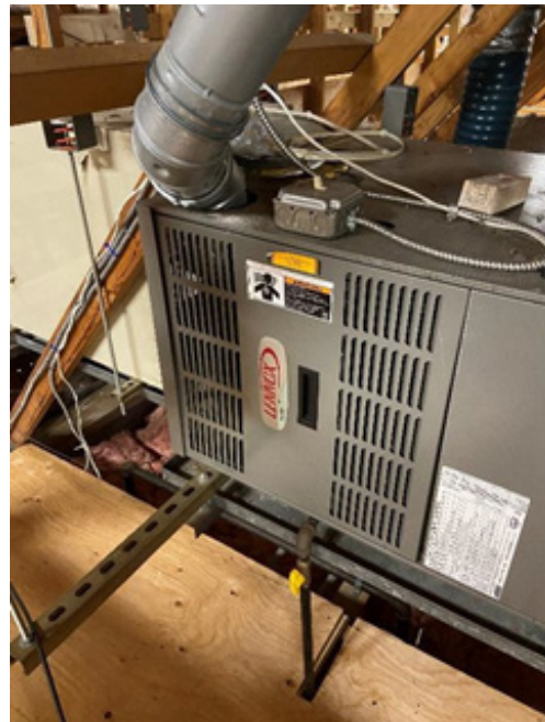
Furnace Unit in Attic Space
