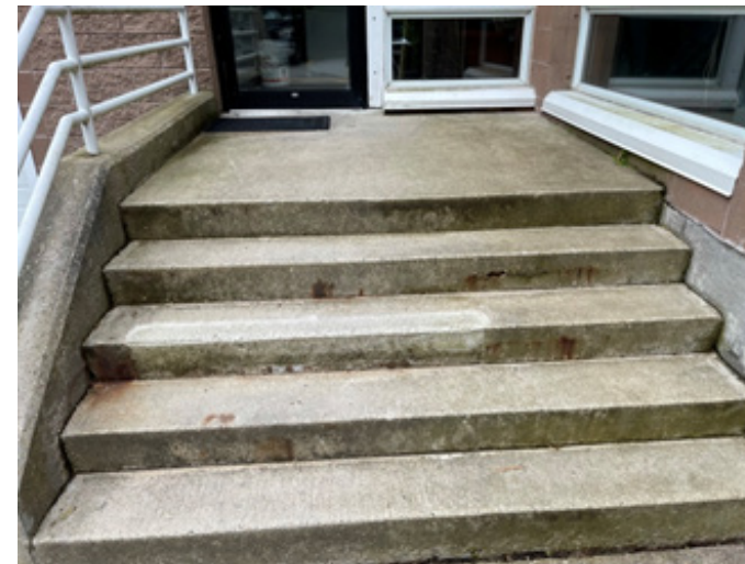
Photo #4 Building West Elevation Concrete steps with minor cracks and surface rusting observed
