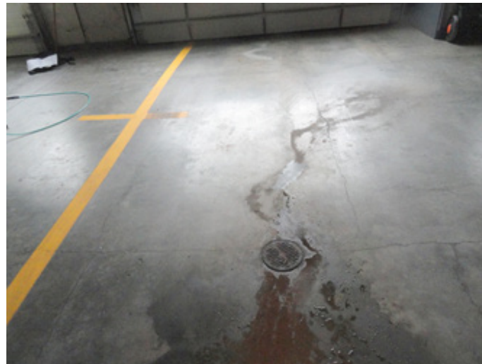
Photo #11 Basement Apparatus Room slab Shrinkage cracks at the front middle bay
